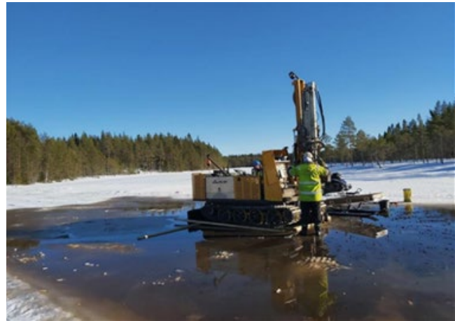
Figure 3. Drilling to Test Till and Bedrock Geochemistry Under a Lake at the Isoneva Project
